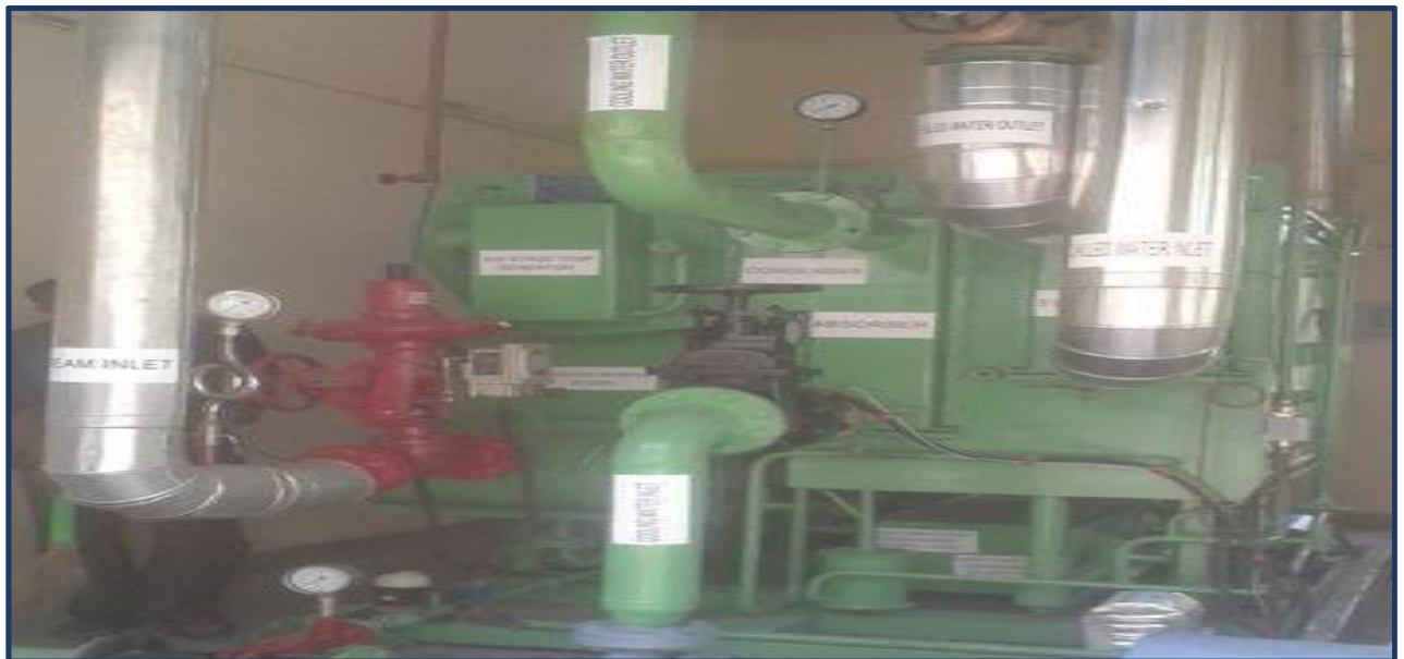
Vapur Absorption Refrigeration Unit at Gokul Dairy, Kolhapur.
